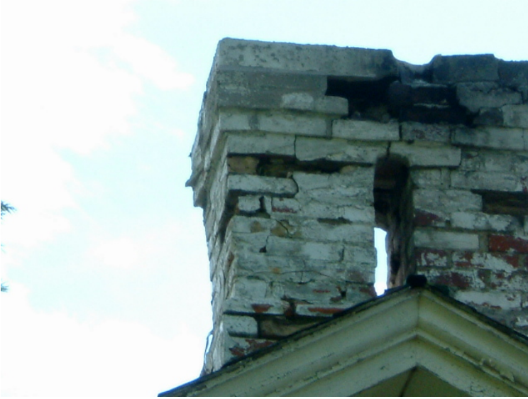
Chimney (Brickwork spalling and missing bricks)
