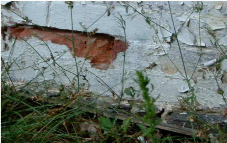
Brickwork Spalling at East Elevation
