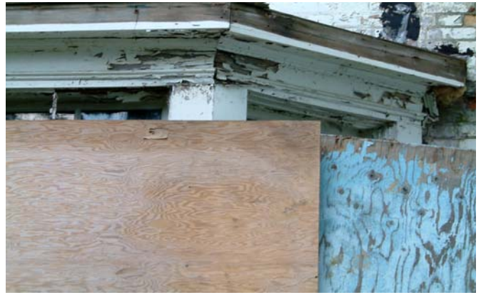
Wood deterioration by water/moisture at east elevation
